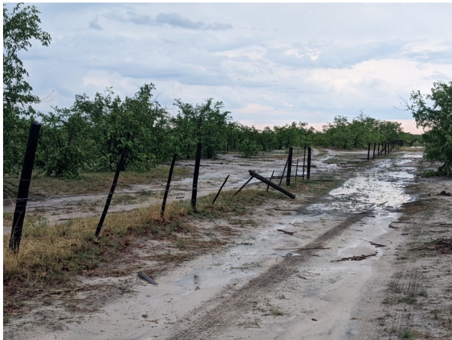
Figure 18. Northern Buffalo fence in poor condition with missing wires and major breaks during a site visit in November 2022.
