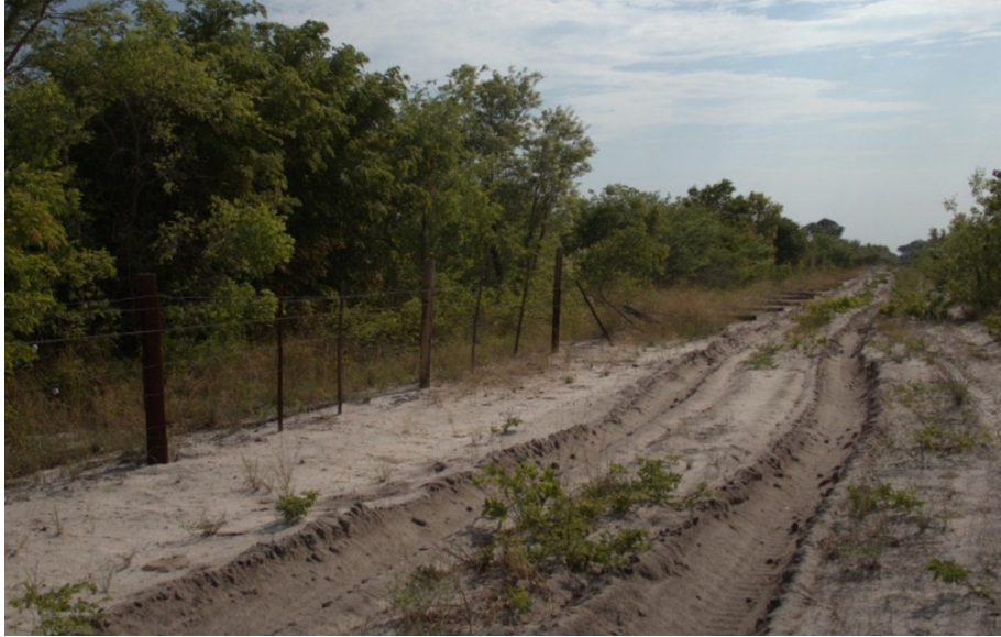
Figure 12. Eastern Zambezi Border fence, showing intact and upright fence posts followed by a section of downed posts and wires during a site visit in November 2022.
